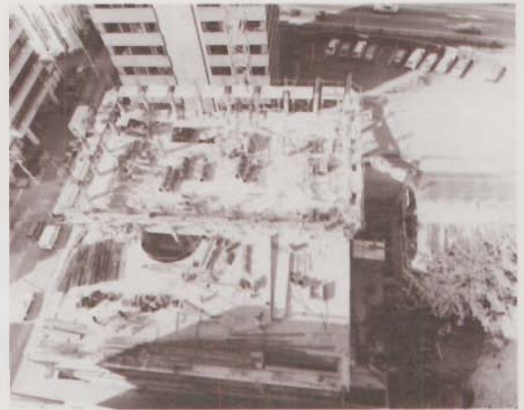
ECOLOGY IN ACTION A 10-story national headquarters for HP New Zealand in Wellington is starting to take shape on the site of the old Victoria Market. Care has been taken to preserve a 200-year-old Norfolk pine and feature it in the rear parking area. Initially HP will occupy three floors of the building which should be ready in December.
